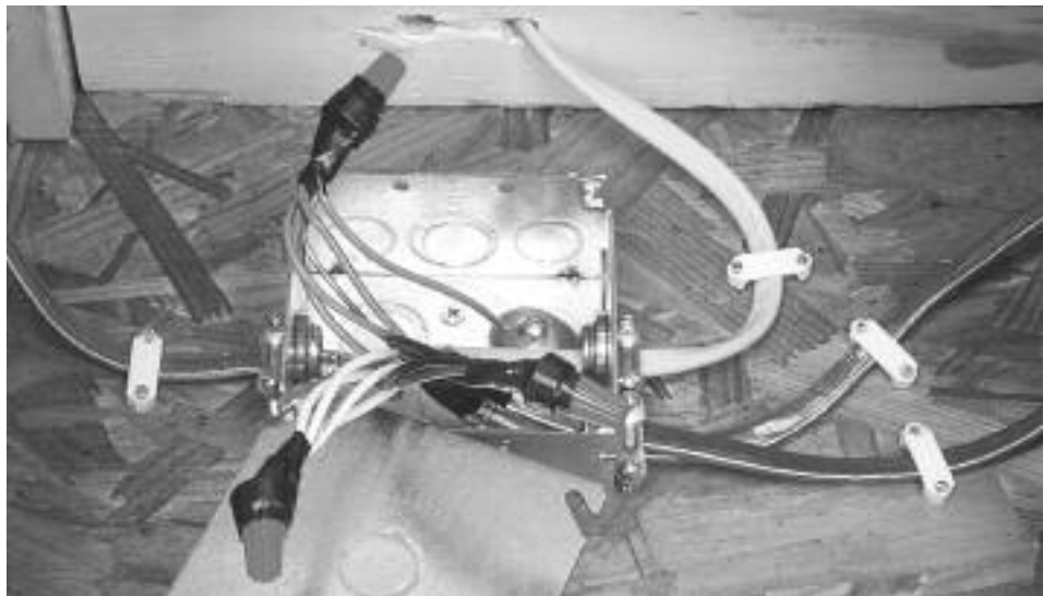
Junction box with multiple sets of mat lead wires, connected in parallel, and connected to the power supply.
