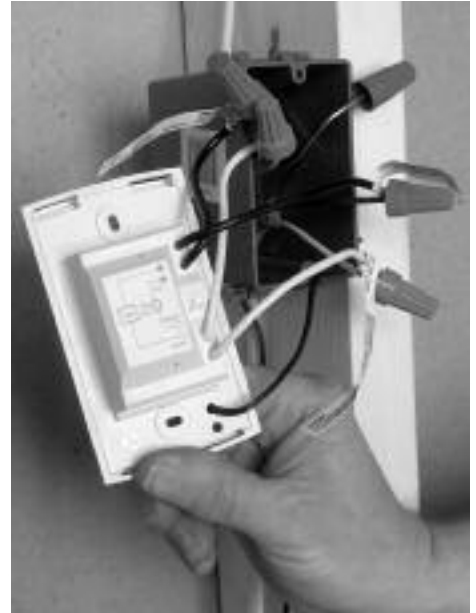
The mat power leads and sensor wire connected to the control at the electrical box.
