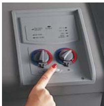
LT Temperature Controls
